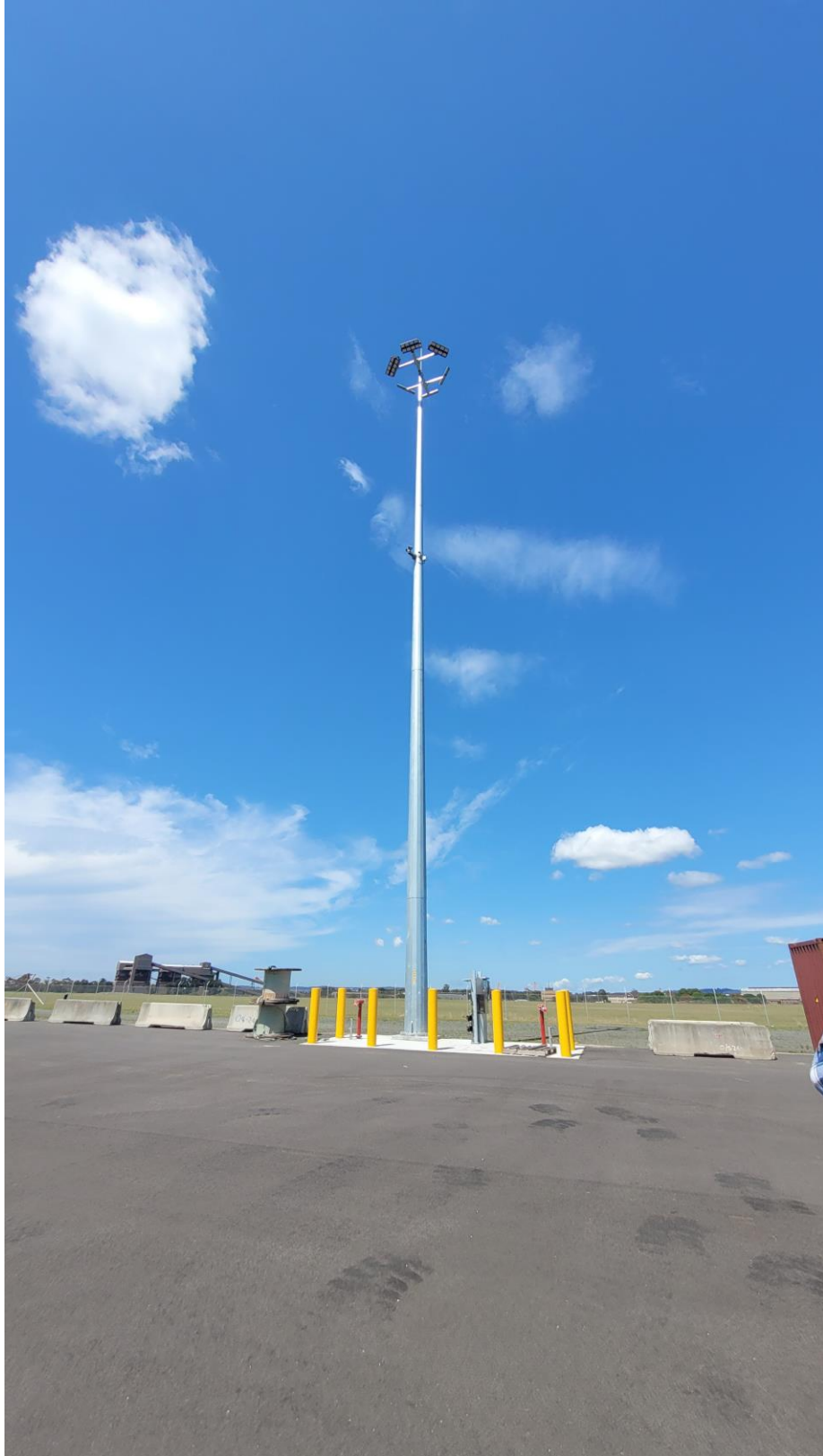
Photo 3: Mayfield 4 Berth new facility lighting
